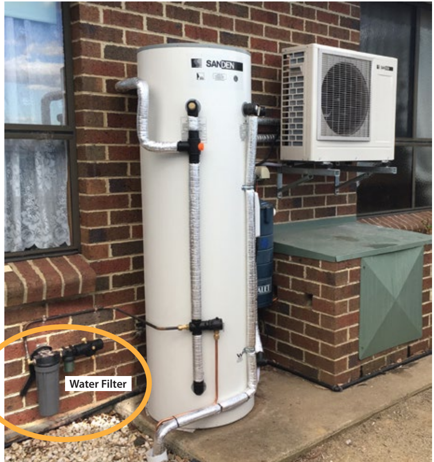
Typical water filter installed
